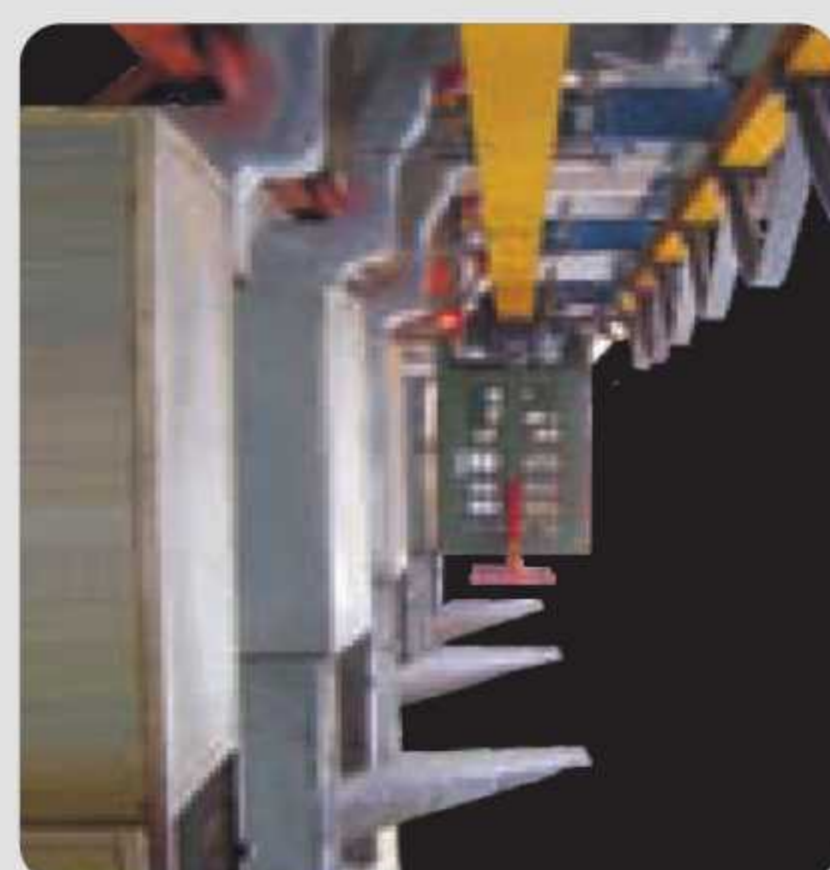
Automatic Portering system (central furnace)
